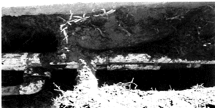
Repaired main line leak on inside loop of Boulevard adjacent from Ring Power.
